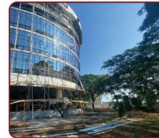
Student Center Building inspection at the TSU Lucinda Campus damaged by a typhoon.
